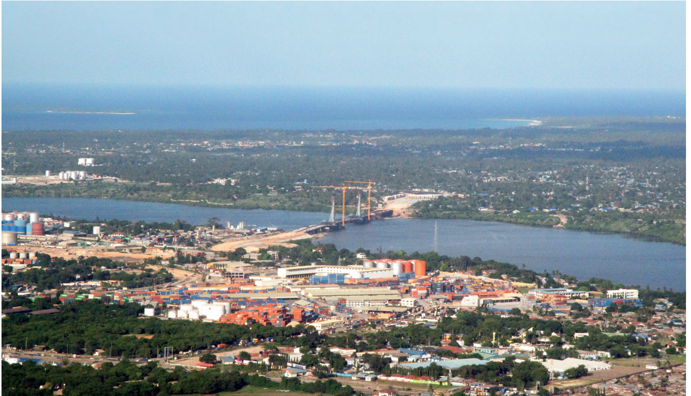
Aerial view of the new Kigamboni Bridge (under construction) connecting Dar es Salaam with Temeke District's southern areas
